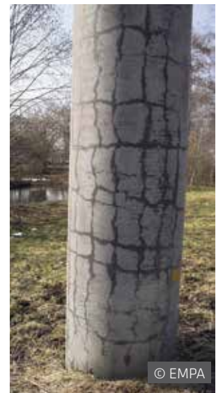
The appearance of ASR damage can be assessed very well on the drying concrete surface of this bridge pylon. Damage can appear within years or only after decades.
