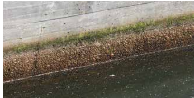
Heavy leaching and damage to the structural concrete are observed particularly in the water splash zone of biological treatment basins.
