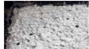
Very severe surface weathering
