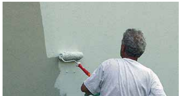
Epoxy resin-based protective coatings are applied over the entire surface following reprofiling of the concrete surface with sulfate-resistant repair mortar enhanced with synthetic material.
