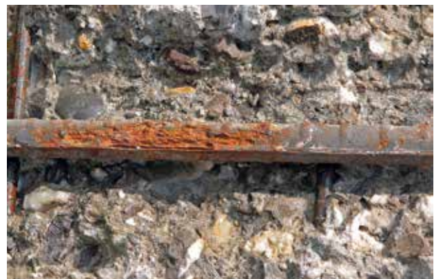
Damage to concrete structure due to insufficient concrete cover and low concrete quality
