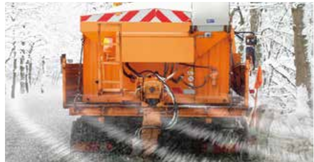
Scattered de-icing agent considerably intensifies the reaction upon freezing of water and leads to substantially greater damage in areas of concrete close to the surface.
