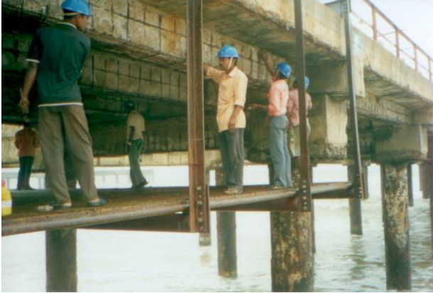
Installation of a temporary hanging truss as working platform to access the underside of the jetty.
